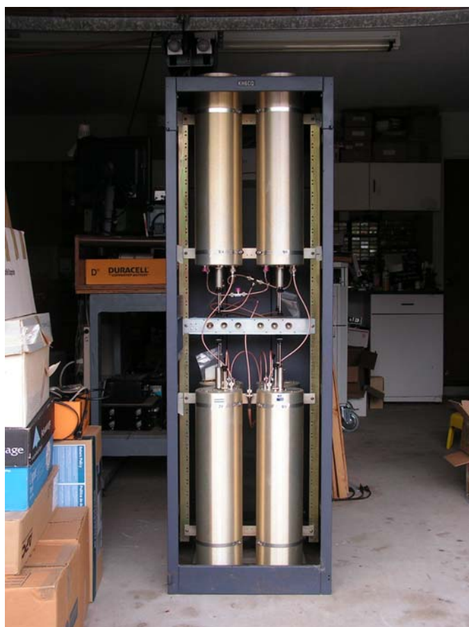
Figure 1 — The two duplexers and band pass cavities mounted in a re-purposed General Electric 19-inch rack cabinet. The front door of the cabinet was removed for this picture.
