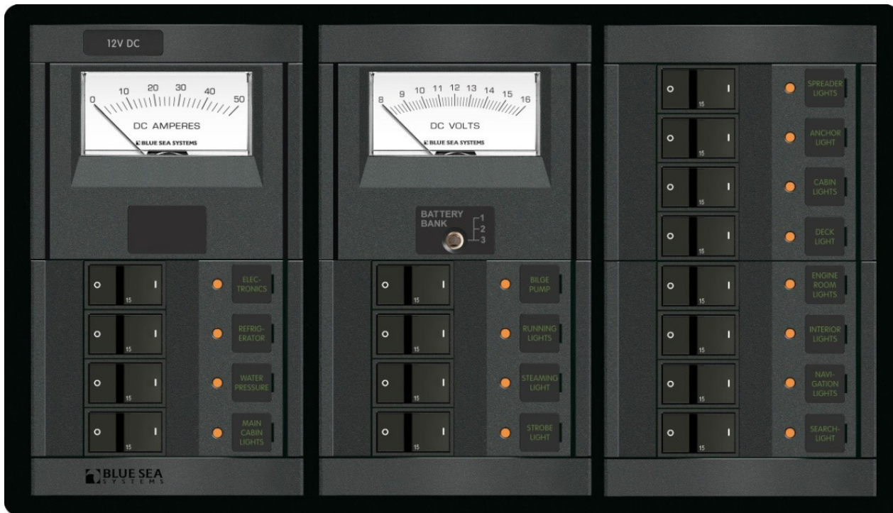
Figure G-44 Example of Marine 12V DC Power Distribution Panel (Photo Courtesy of Blue Sea Systems)
